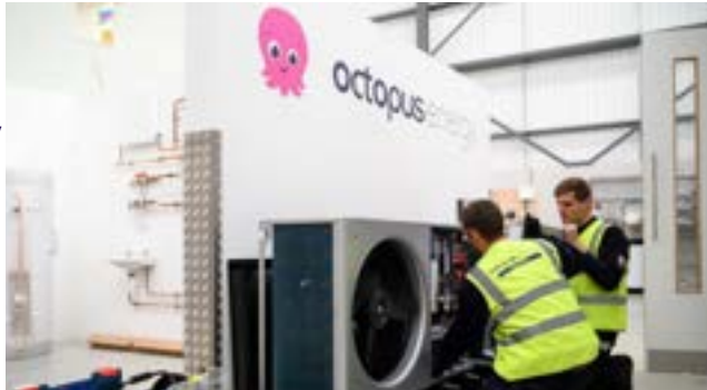
Low carbon tech installation
